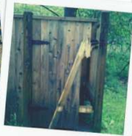
bear damage outhouse
